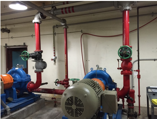
Figure 9. Deluge system firewater pumps
