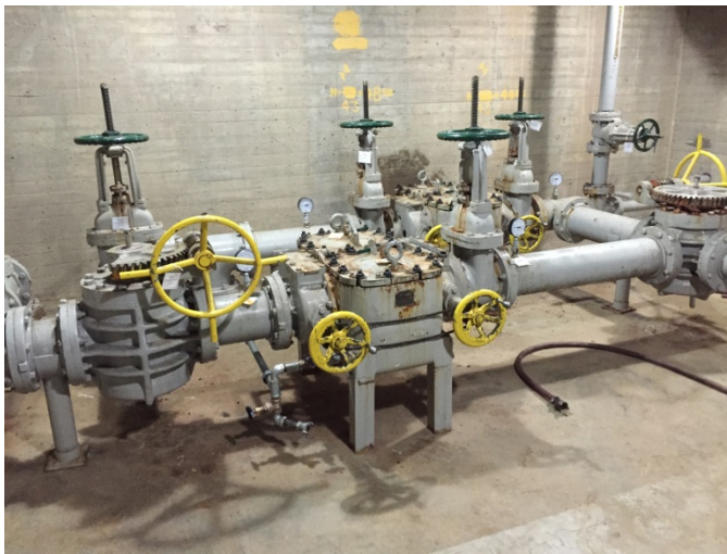
Figure 6. Cooling water system duplex strainers
