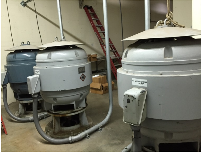
Figure 12. Unwatering sump pumps
