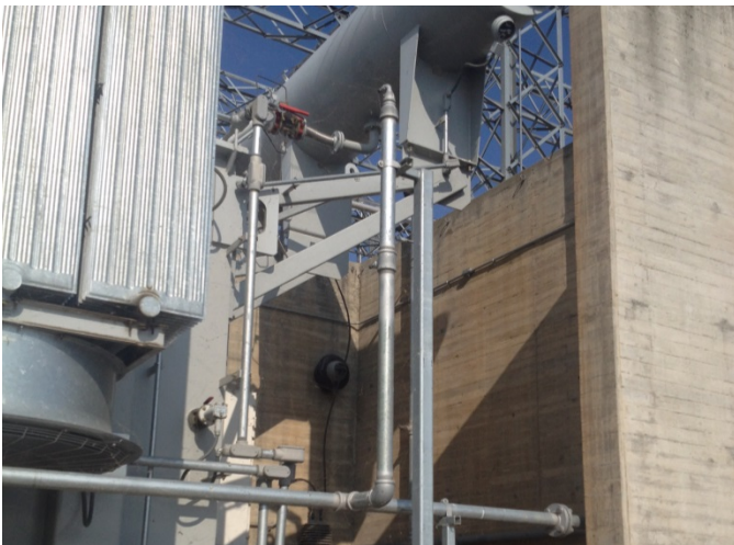
Figure 10. Transformer deluge system distribution piping and nozzles
