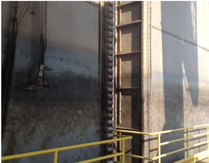
Figure 5. Roller gate and bulkhead gate
