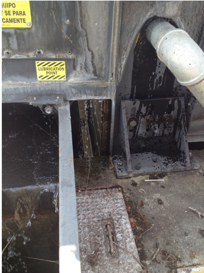
Figure 14. South intake traveling water screen spray water supply
