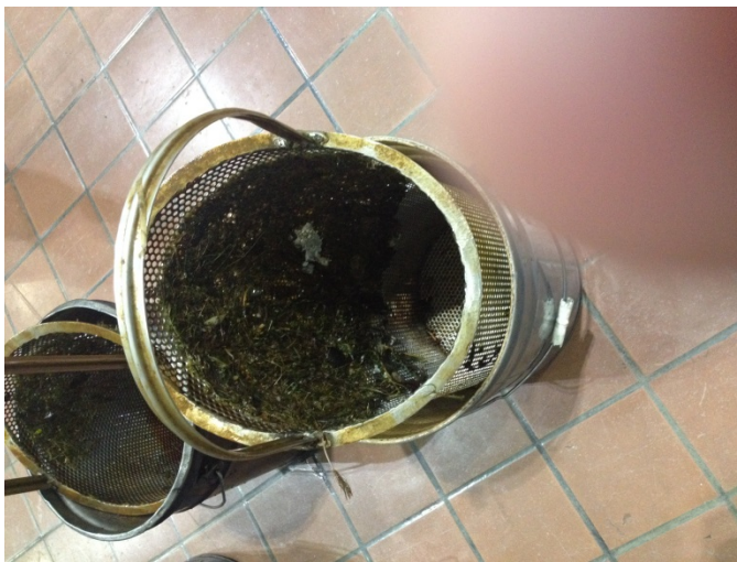
Figure 7. Cooling water strainer baskets
