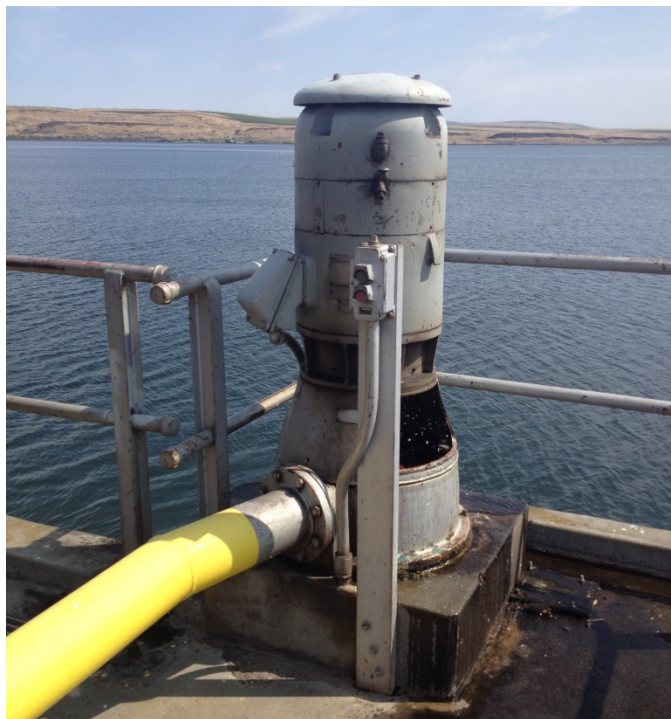
Figure 15. Traveling water screen wash supply pump
