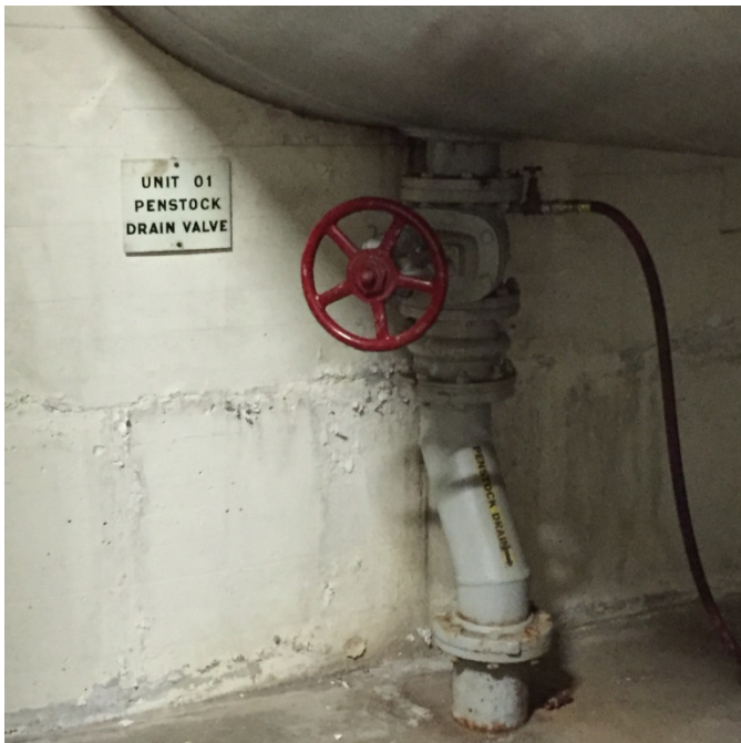
Figure 11. Station power penstock drain
