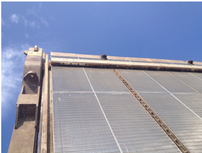
Figure 4. Intake screen panels and brush system
