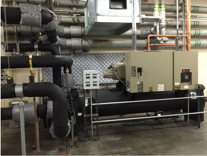
Figure 8. Oil cooler heat exchangers
